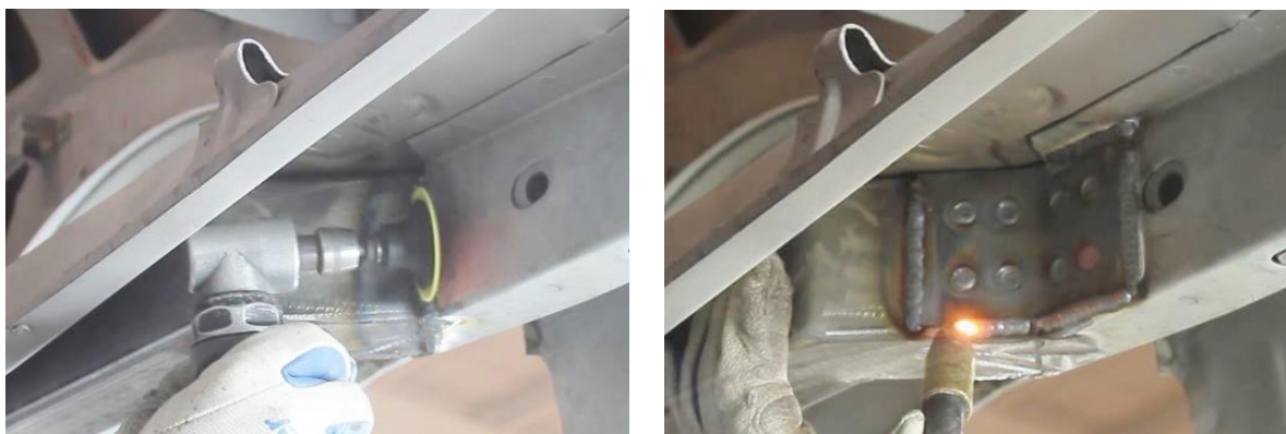
Figure 23 - Weld Inside Frame Rail Doubler Plate
