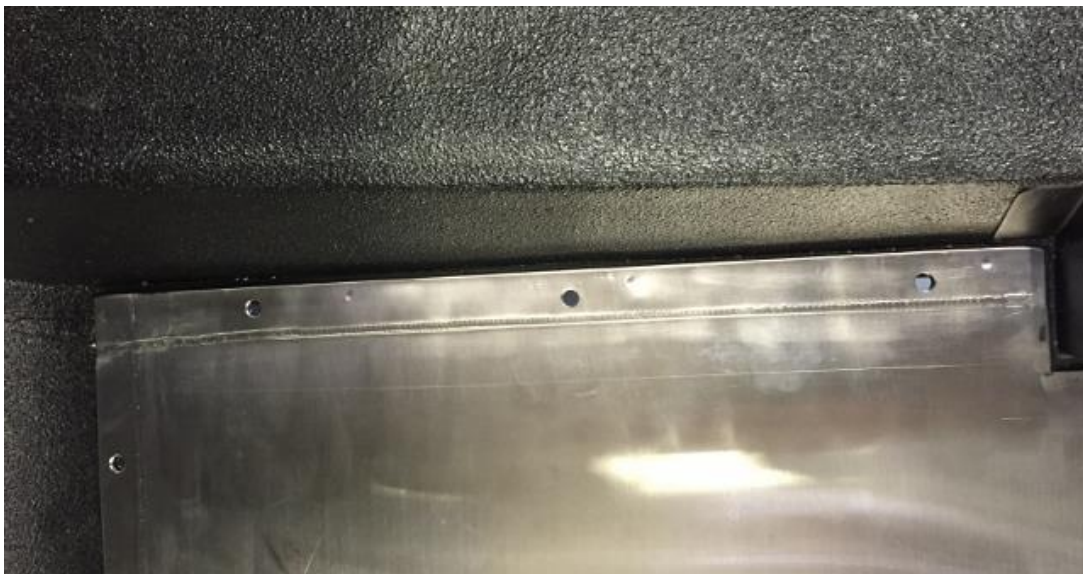
Figure 5 – Drilled Holes in Fuel Tank
