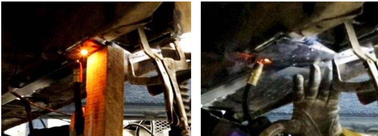
Figure 50 – Weld Doubler Plate
